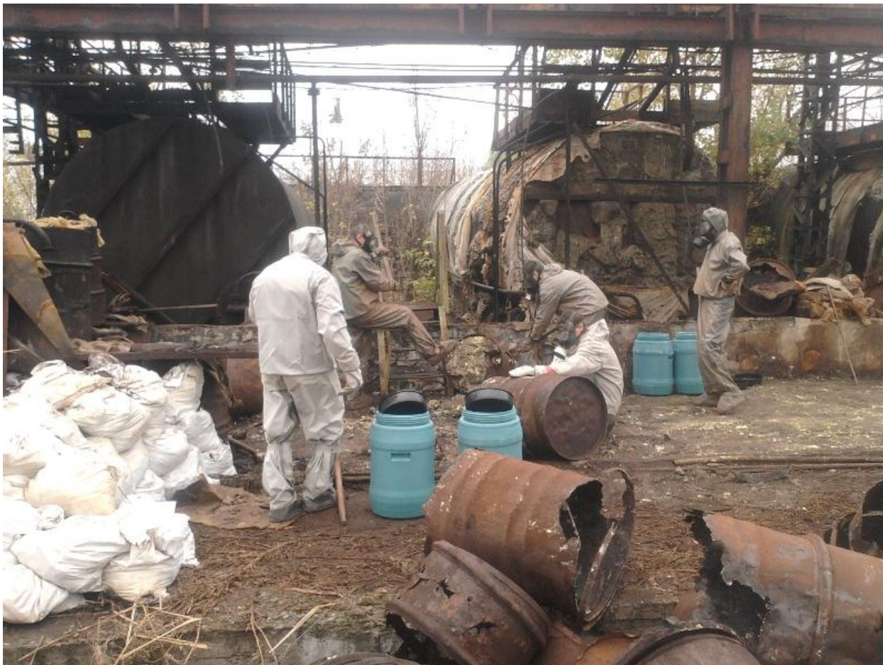
Figure 2 Collecting MNCB containing waste in Gorlovka
